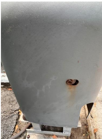
Access point for override crank
